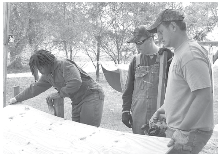
Craig R-3 seniors, Kyree Howell, Zach Marks and Jacob Dougherty, left to right - Work to repair a deck for an elderly woman in the Craig, MO, community. Students at Craig R-3 completed a community volunteer project on Thursday morning, October 22, before an early dismissal for parent-teacher conferences.
