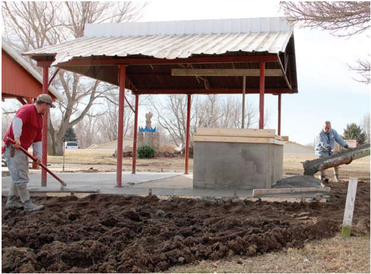
(Left) New cement was the first of the work- That was being done at the fire pit at Griffith Park on Thursday, February 23. Gordan Gallandt (right) and Michael Selleck (left) of Mid-American Restoration, LLC, were awarded the bid for the project by the city of Mound City.
