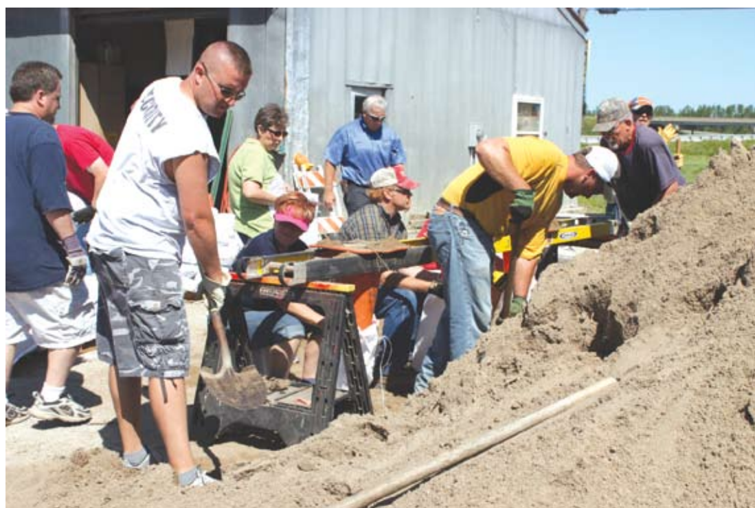
Both manual sandbagging (above)- And mechanical sandbagging by as many as 30 volunteers helped fill nearly 8,000 sandbags to be used in or near Mound City in its fight against the encroaching floodwaters that are making their way toward town. Sandbags were hauled to low sections on the north side levee of Davis Creek to help ensure the creek stays in its bank should it rise again from either floodwaters backing up or from rapid rainfall as seen in the community this past weekend. Pallets of sandbags now stand at the ready to be used to complete the project and potentially ward off flash flood rainwater at Evans Circle. More sandbags and levee work will take place today, Thursday, June 30.
