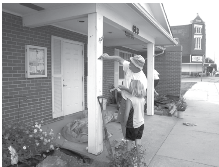
Dennis Reule, left, and Daniell Brandon, right- Are pictured above preparing to paint the Nutrition Site in Mound City. Along with other VBS students from the First Christian Church in Mound City, they worked all week weeding, planting, painting and cleaning up around town.
