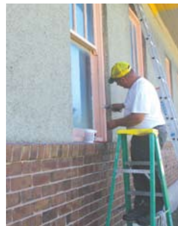
The Mound City Depot Museum- Is getting a fresh coat of paint by Jeff Weedin of Fairfax, MO. He is pictured caulking the windows that have already been primed for new paint. The eave, pictured above, has been partially painted with the taupe (pictured at the back) primer. The stucco (sides) and the brick are historically the exterior of depots of the 1920 era.
